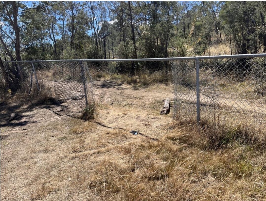
Figure A4-8: Existing hole in fence
