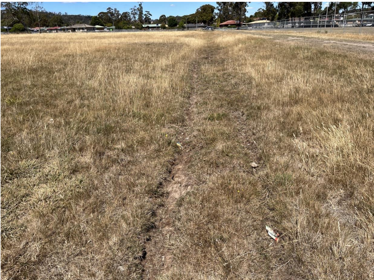
Figure A3-4: View south east along the drain in the west of the title.
